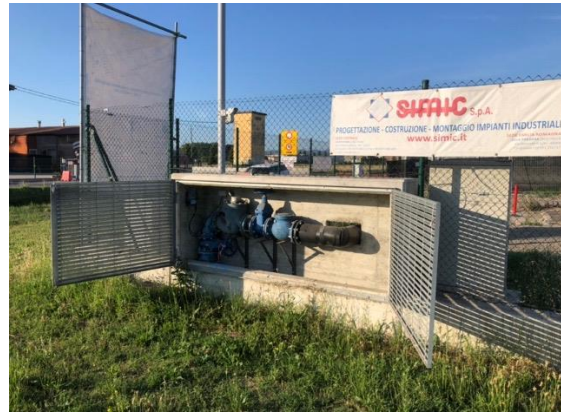
Inlet water point
