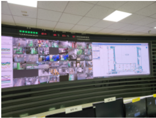
Real-time monitoring data at control room [SecuCam]taewoan.koo@samsung.com_20221107101432.jpg
