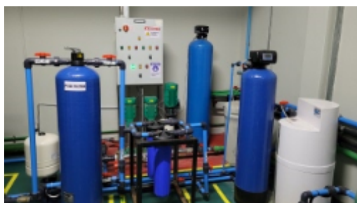
Utilities Area domestic water treatment back-up system 2.jpg
