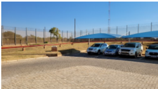
BAT above ground water pipeline.jpg
