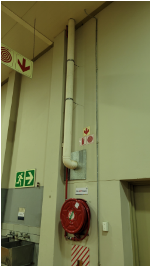
Fire suppression system in factory.jpg
