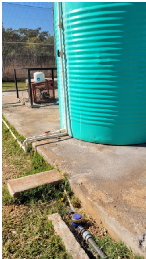
Site Change Room water storage tank and pump.jpg
