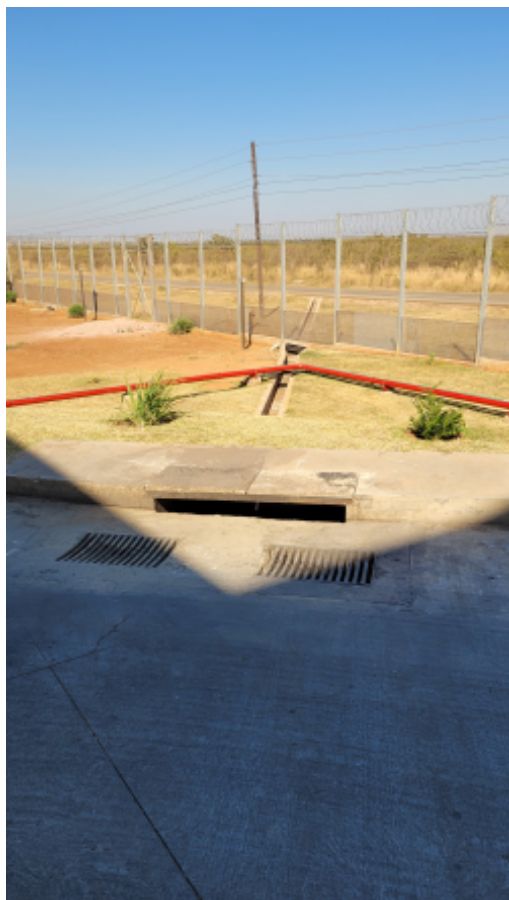
Stormwater system on site.jpg
