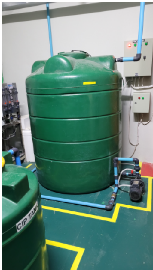
Utilities Area domestic water treatment back-up system 4.jpg
