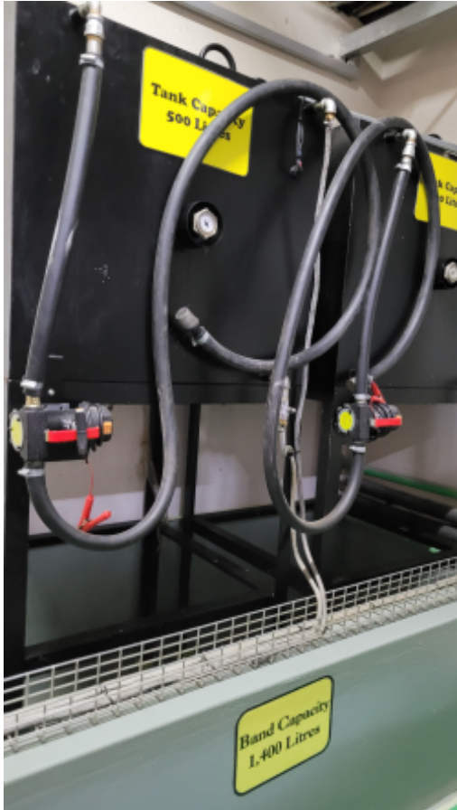
Utilities Area fuel storage tanks with bunding.jpg
