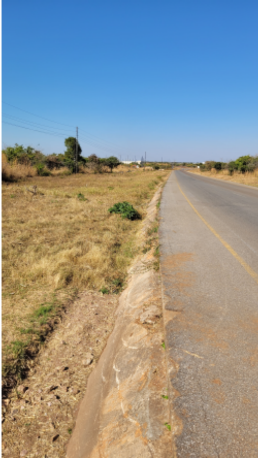
MFEZ stormwater system downstream of the site..jpg
