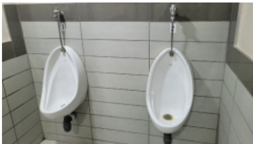
Office restroom urinal.jpg
