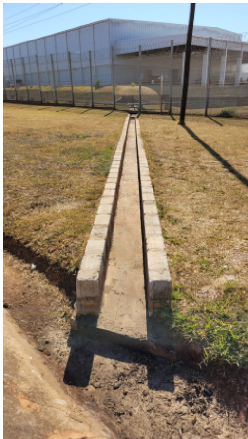
MFEZ stormwater system from the site 2..jpg
