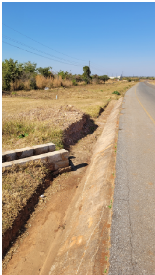
MFEZ stormwater system from the site.jpg
