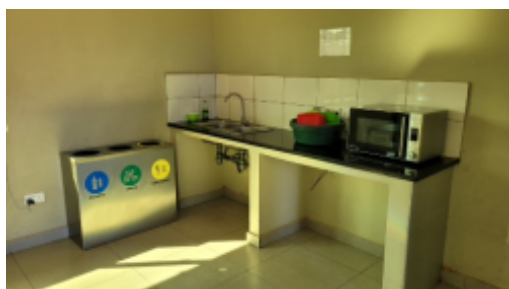
Site Change Room kitchen basin.jpg
