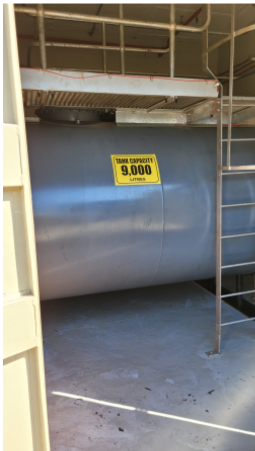
Bunded diesel storage tank.jpg
