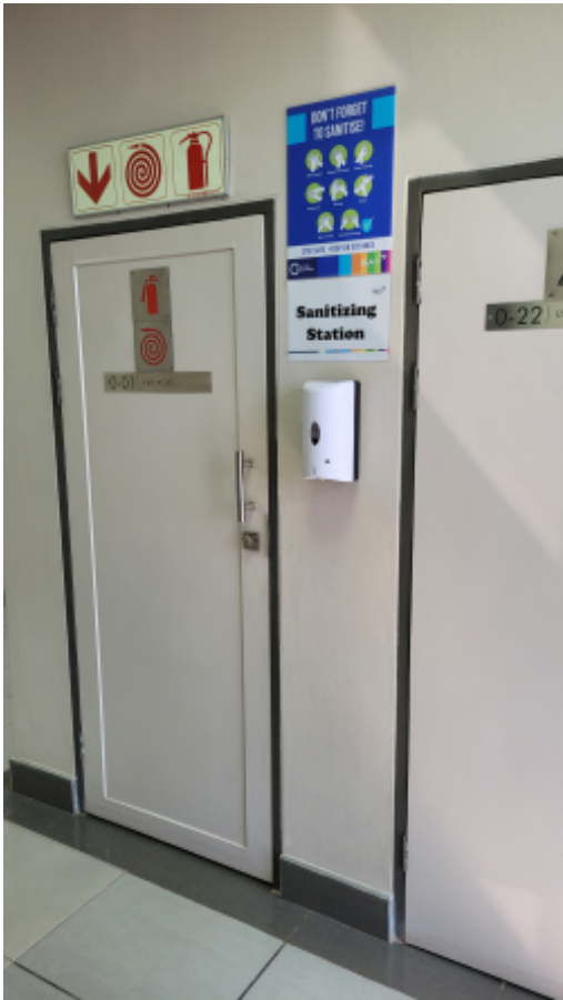
Utilities Area sanitation station.jpg
