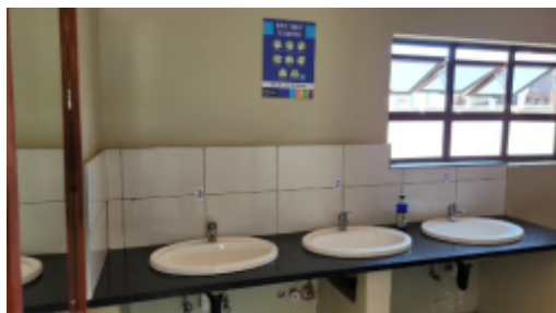
Site Change Room restroom basins.jpg
