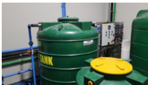
Utilities Area domestic water treatment back-up system 3.jpg
