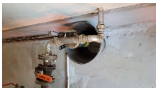
Water line valve leak awaiting repair.jpg
