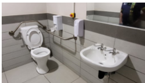
Office restroom disabled toilet and basin.jpg
