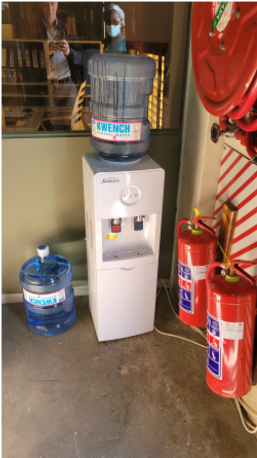
Utilities Area drinking water station.jpg
