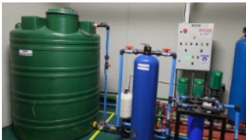
Utilities Area domestic water treatment back-up system.jpg
