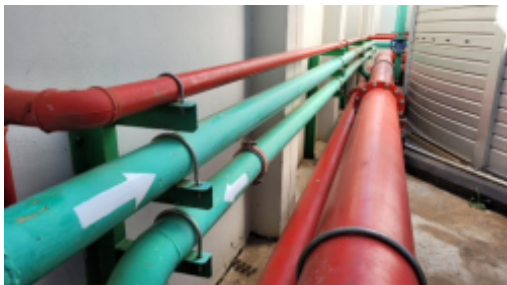
Site pipeline to storage tanks.jpg
