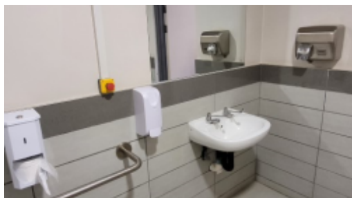
Office restroom disabled toilet and basin and hand dryer.jpg
