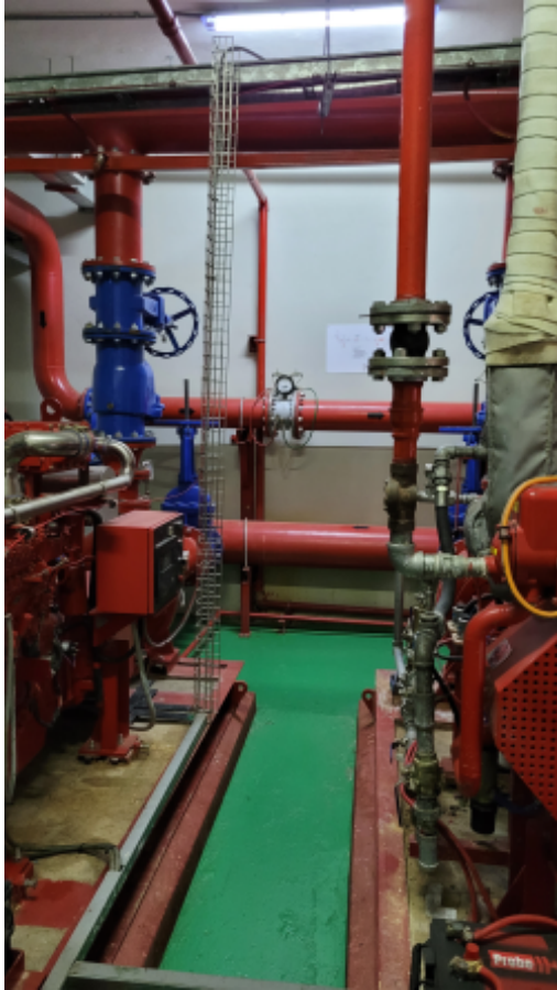
Utilities water pumps and meters.jpg
