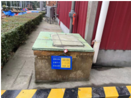
Initial rainwater collection pond-Furong Plant.jpg
