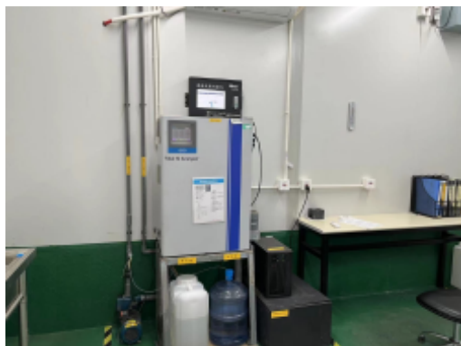
Online monitoring facilities-Furong Plant (1).jpg
