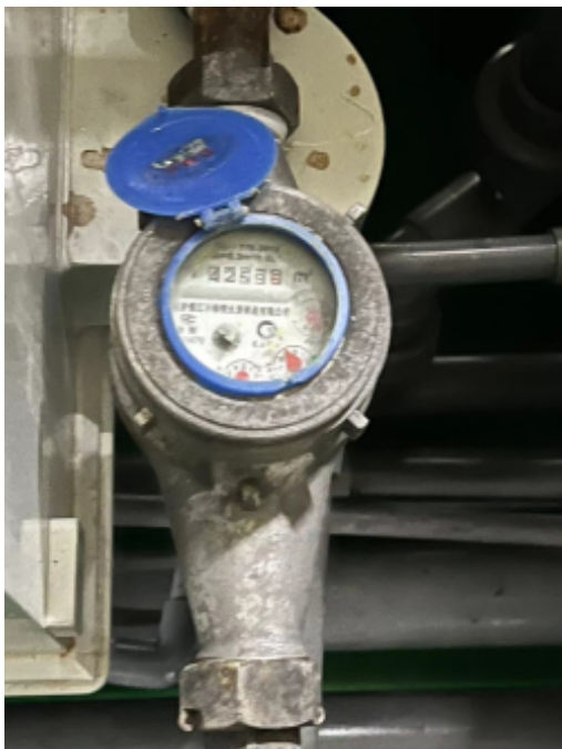
Water meter-Furong Plant.jpg
