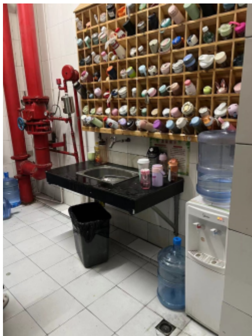
Drinking water area-Furong Plant.jpg
