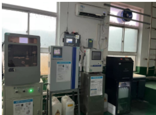
Online monitoring facilities-Furong Plant (2).jpg
