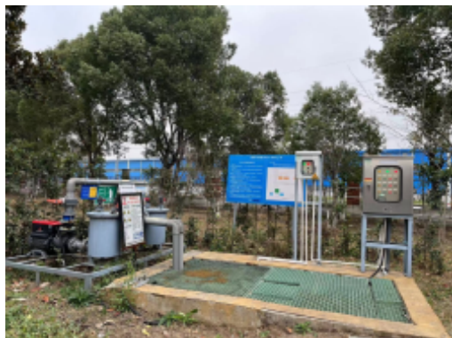
Rain water discharge point-Furong Plant.jpg
