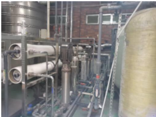
Drinking water-Tuanjie Plant.jpg
