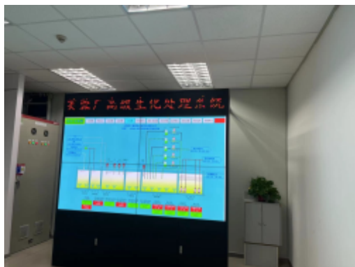
Wastewater intelligent monitoring platform.jpg
