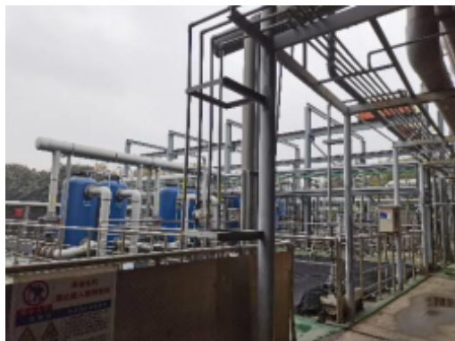
Wastewater treatment-Tuanjie Plant (2).jpg
