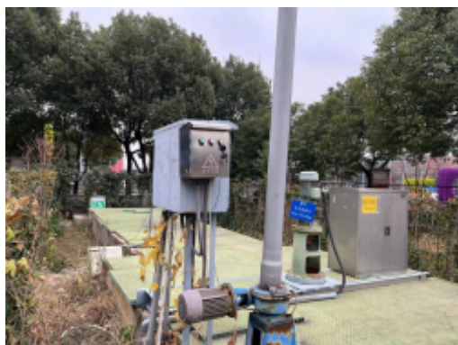
Industrial wastewater discharge point-Furong Plant.jpg
