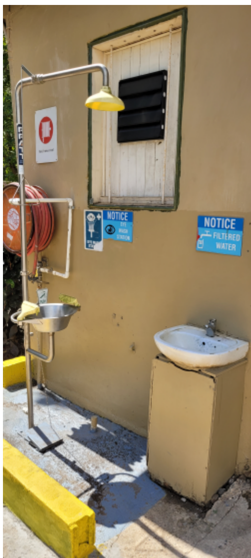
Eye wash station outside chemical store.jpg
