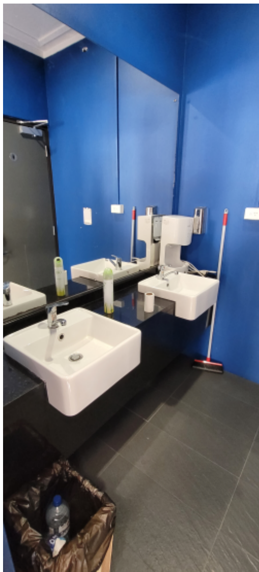
Handwash basins at marketing department bathroom.jpg
