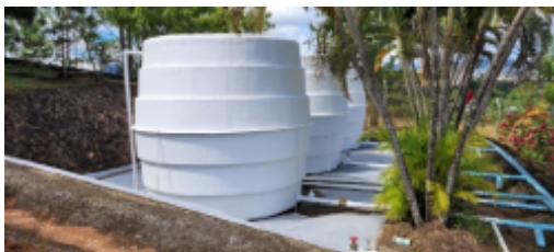
Water Storage Tanks.jpg
