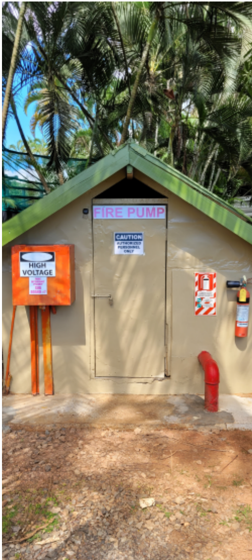
Fire suppression pump house.jpg
