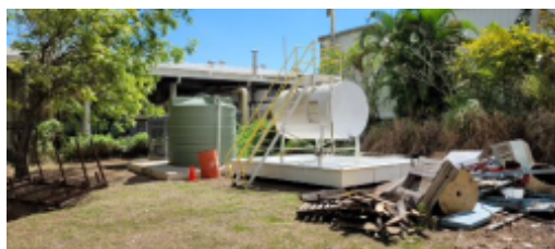
Fuel Storage Tank and Water Storage Tank outside GLT plant.jpg
