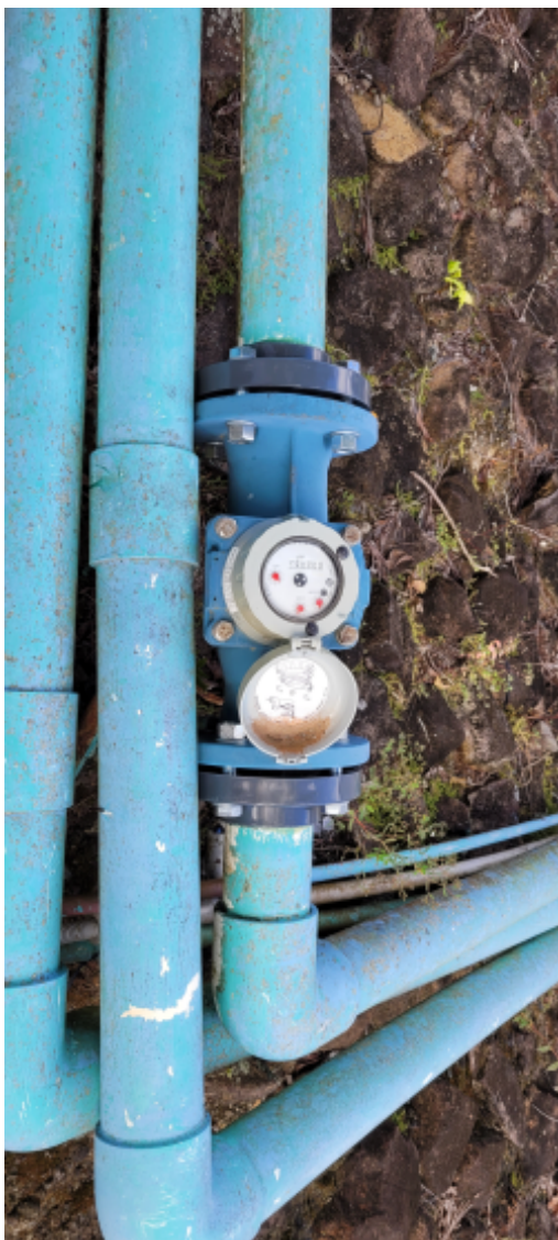
Metering for Water Storage Tanks.jpg
