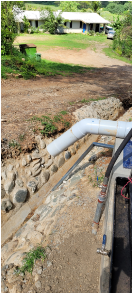
Stormwater system adjacent to new boiler.jpg
