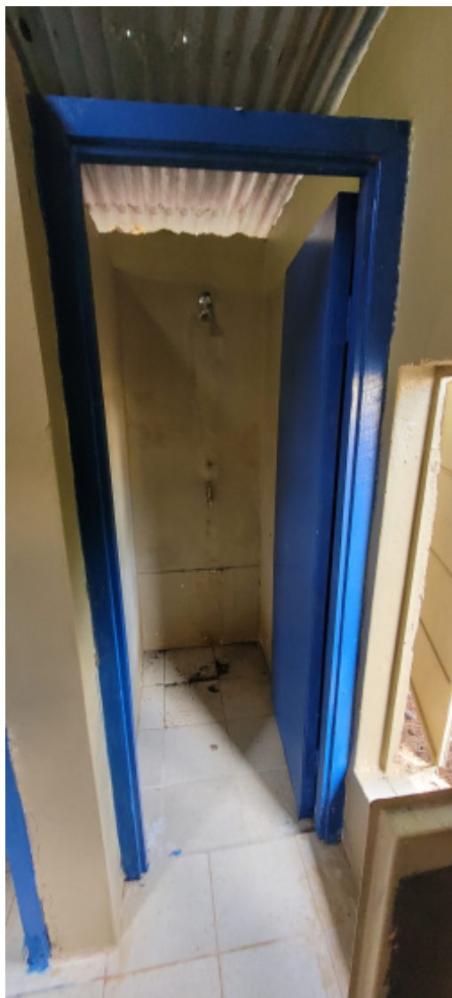
Shower near mechanical maintenance area.jpg
