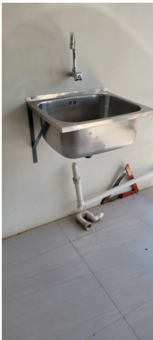
Handwash basin outside marketing offices requiring minor maintenance.jpg
