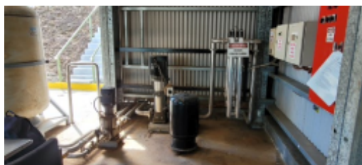
On-site borehole pump.jpg
