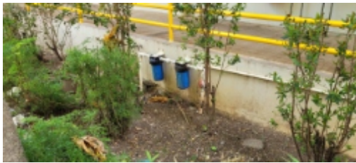
Newly installed water filters.jpg
