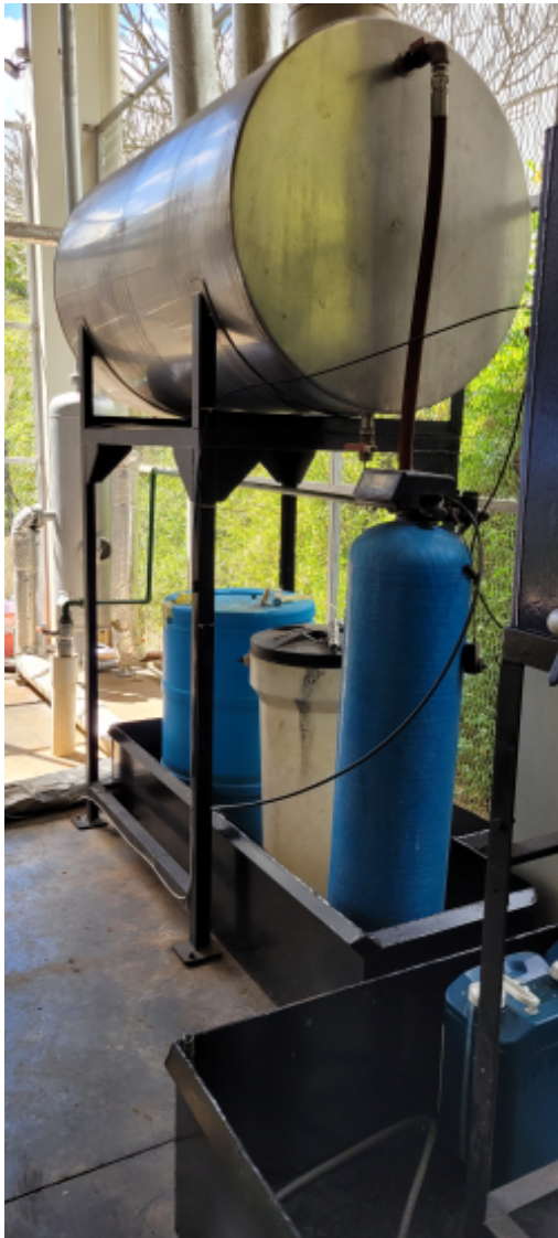
Bunded chemicals at GLT Plant.jpg
