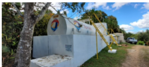
Diesel storage tank with bunding.jpg
