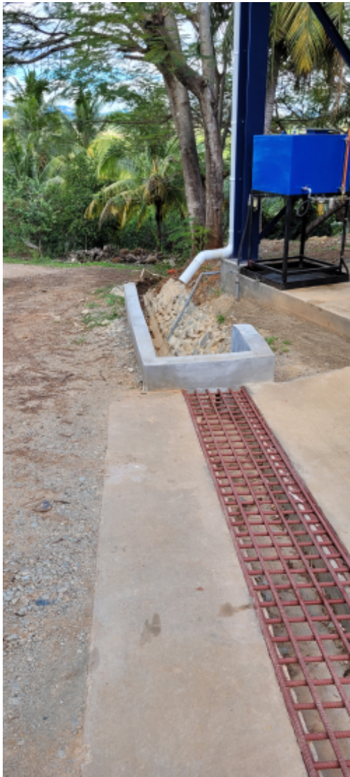
Stormwater drain at new boiler.jpg
