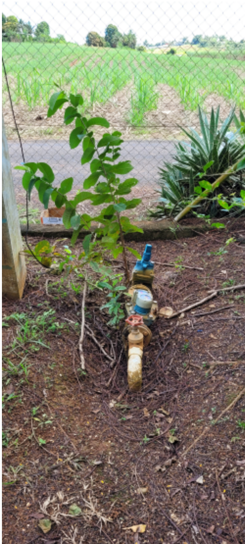
WAF meter for input water to the site.jpg
