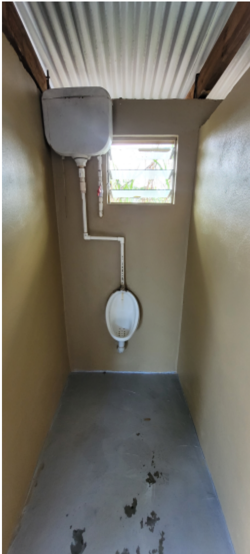
Urinal near Water Storage Tanks.jpg
