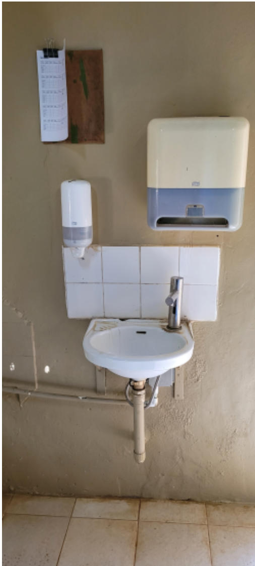
Handwash basin in bathroom near mechanical maintenance area.j.jpg
