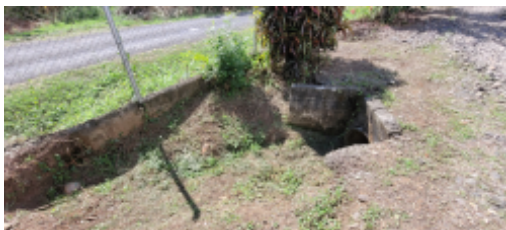
Stormwater system leaving site on western site boundary.jpg
