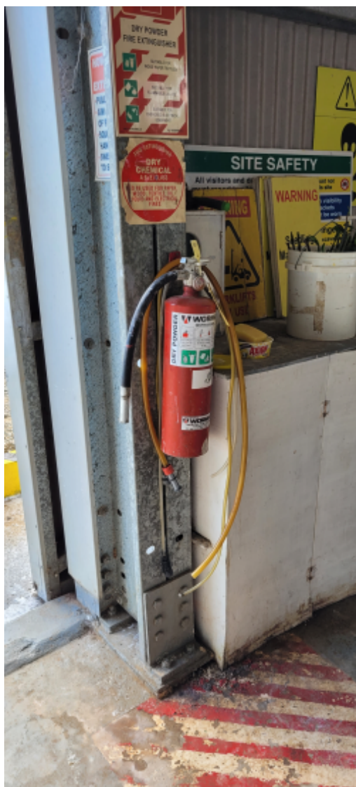
Fire extinguisher (non-water based).jpg
