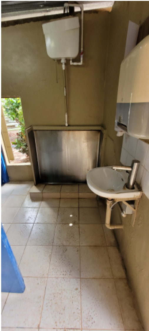
Urinal and handwash basin in bathroom near Mechanical maintenance area.jpg
