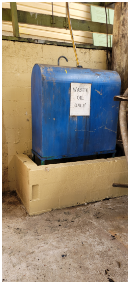
Use oil storage container prior to disposal in Mechanical maintenance area.jpg
