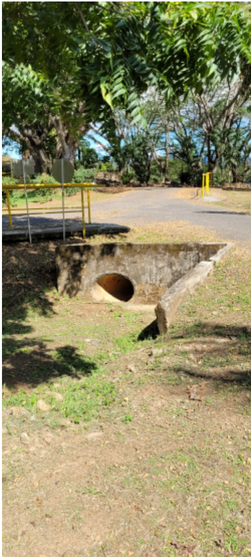
Stormwater system near site entrance and exit point.jpg
