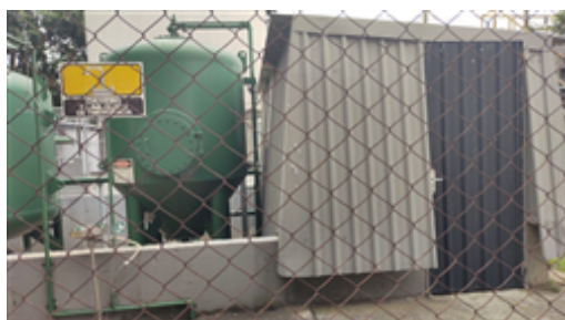
Water treatment plant, filtration and addition of sodium hypochlorite.jpeg
