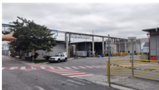
Utilities area with boiler, nitrogen tank and CO2 tank (for mineral water gasification).jpeg
