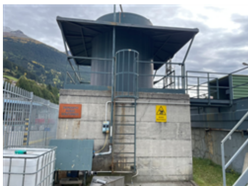
9 chemical storage at waste water section.jpeg
