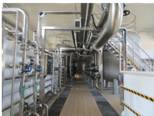
water treatment system.JPG
