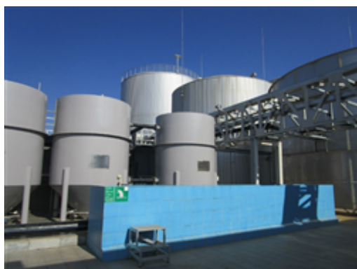
waste water treatment station.JPG
