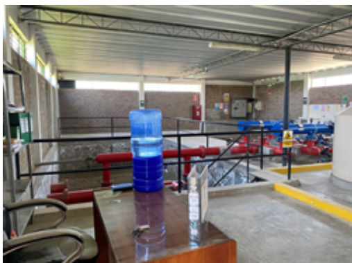
Irrigation and fertigation room - Don Lito Farm IMG_3687.jpg
