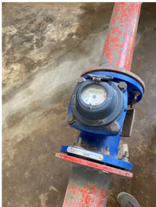
Flowmeter of the Ramón subway well in the Guerrero farm.
