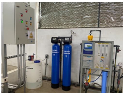
Drinking water treatment Reverse osmosis reverse osmosis Guerrero farm IMG_3306.jpg
