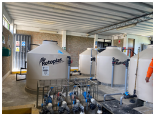
Irrigation and fertigation room - Don Lito Farm
