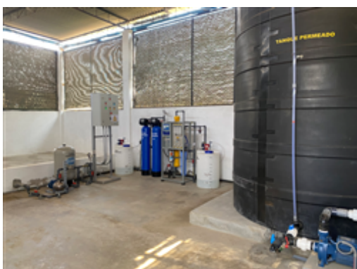
Drinking water treatment Reverse osmosis reverse osmosis Guerrero farm IMG_3304.jpg
