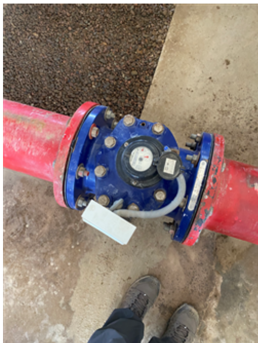
Fundo Guerrero - Flowmeter in irrigation and fertilization room. IMG_3325.jpg
