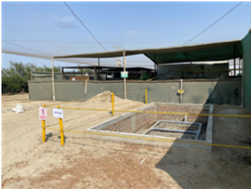
Industrial wastewater treatment system-Biocama Don Gonzalo Farm IMG_3545.jpg
