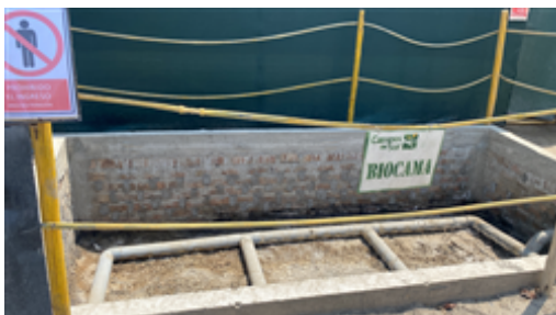
Biocama: Wastewater treatment - Fundo Tronquitos. D696AD1C-E51F-4BAA-8A98-4662B80B1E5A.JPG
