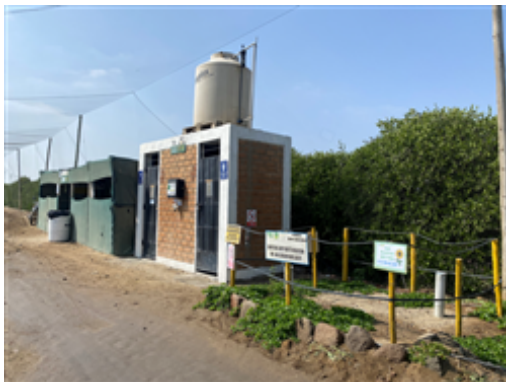
Don Gonzalo Farm Wastewater Treatment System. IMG_3525 (1).jpg
