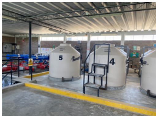
Irrigation and fertigation room - Don Lito Farm IMG_3686.jpg
