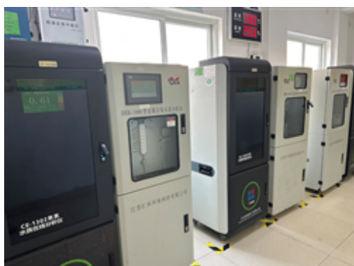
Online wastewater monitoring system.JPG
