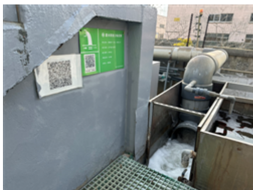
Industrial water discharge point.JPG
